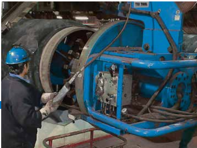
Tri Tool's powerful PIPEMASTER PFM 3248 is being positioned into the end of a concrete lined pipeline section prior to performing weld end preparation.
