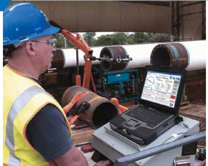
Tri Tool's Laser Dimensioning System records precise measurements of each pipe end so that ends can be accurately matched for improved welding results.
