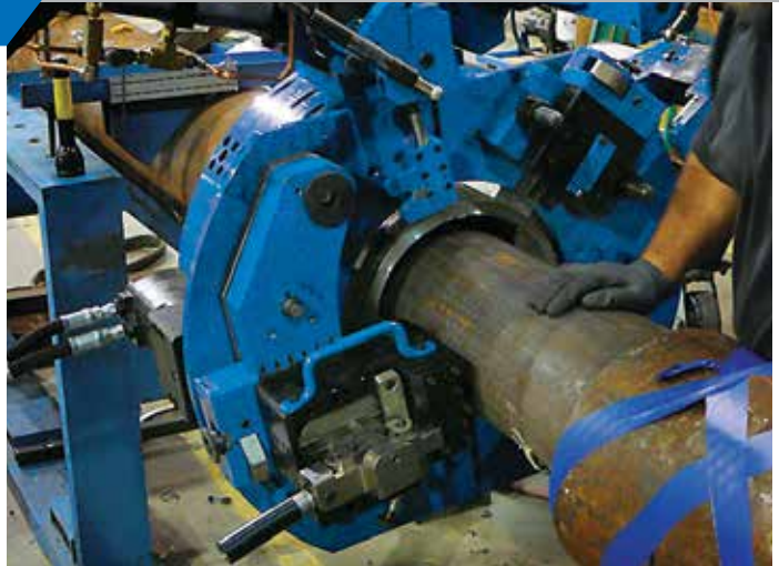
A custom manufactured Clamshell based High Speed Sever System precisely bevels an outer pipe without disturbing the inner pipe.
