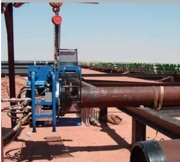
The mission critical nature of end preparation is portrayed by this PFM 816, hard at work in the hot desert sands of Oman on a major land-based pipeline project.
