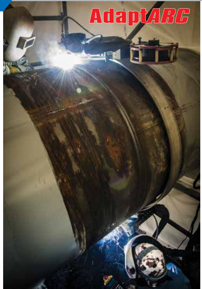
Two Tri Tool DualARC orbital weld heads operating simultaneously on a single mounting track for maximum weld deposition on an onshore LNG project.
