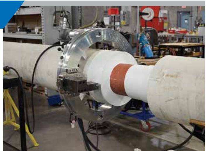
This section of offshore coated pipe is having the coating removed with an in-line, OD mounted TRIMAX split-frame lathe utilizing form tooling.
