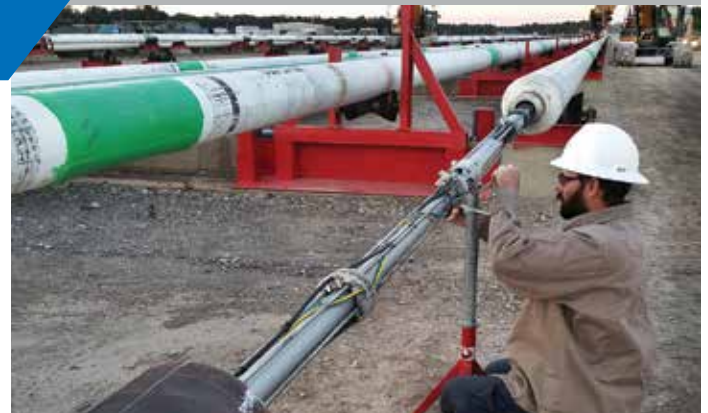
A Tri Tool custom built internal clamp was designed to provide 2D imaging, 3D laser surface inspection, along with precision welding alignment.
