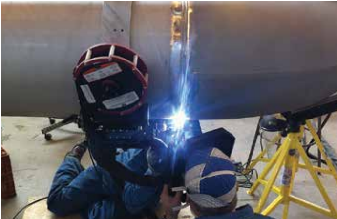
Tri Tool welding technicians performing specialized welds on highly corrosion resistant super duplex stainless steel pipe for a geothermal project.
